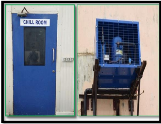
Chill room facility
