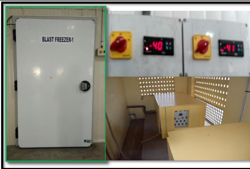
Blast Freezer Facility
