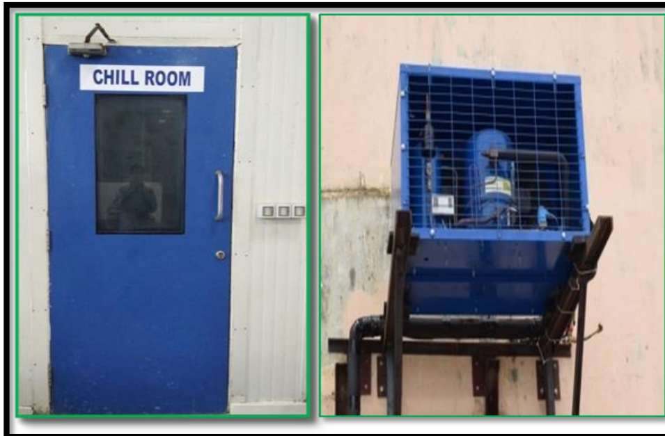
Chill Room Facility
