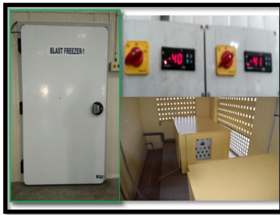
Blast freezer facility
